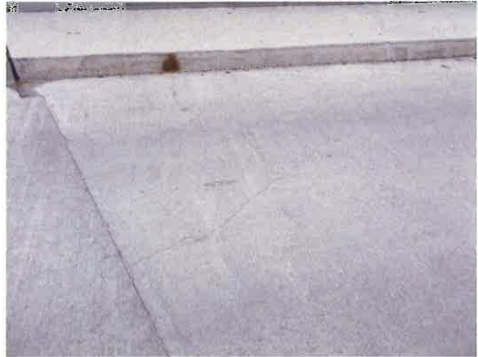
Document Name: DSCN0416.JPG Category: Deck Comments: Diagonal cracks
